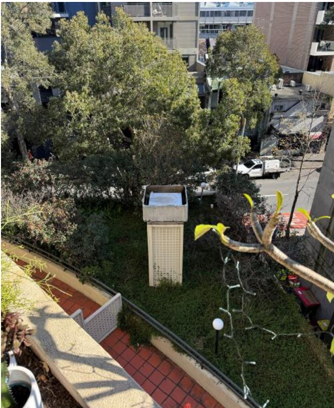
Figure 6: Mechanical exhaust vent for the premises, which is close to residential apartments, looking west towards Elizabeth Street
